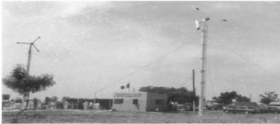
Fig 6: 5KW Wind Power for Village Electrification, Sayya Gidan Gada, Sokoto State Built by SERC
