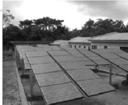
Solar PV at Ilaje, Ondo State of Nigeria
