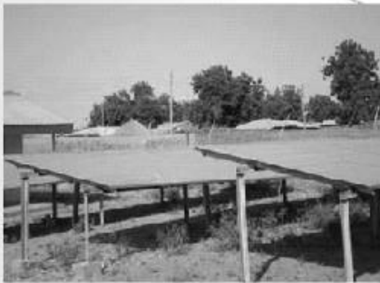
Solar PV mini-grid in a village in Sokoto, Sokoto State
