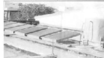
A 1000-litre Solar Water Heating System at the Maternity Ward of Usmanu Danfodiyo University Teaching Hospital, Sokoto constructed by SERC.
